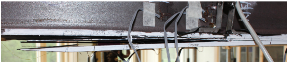
Figure 64: Failure of beam 33, seen from the back.
