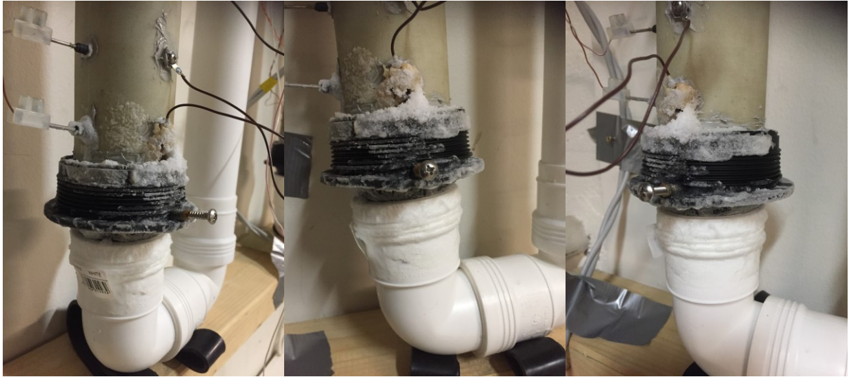
Figure 6-1 Salt migration due to leakage at the lower rubber socket for cylinder A (27.05.2016).
