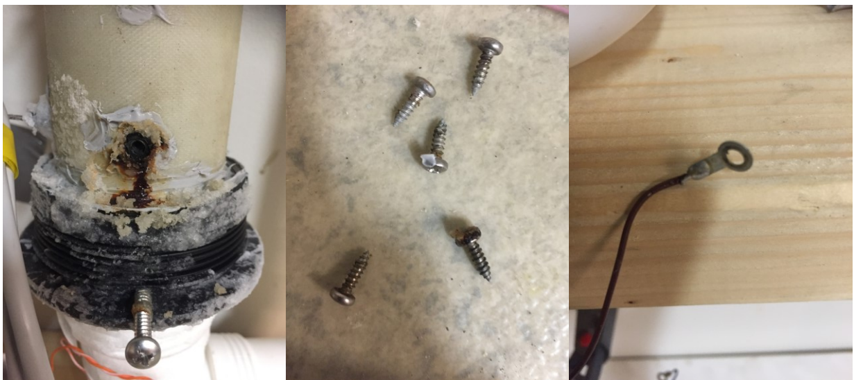
Figure 6-2 Corrosion from the bolt nut, the unaffected screws and coupling.
