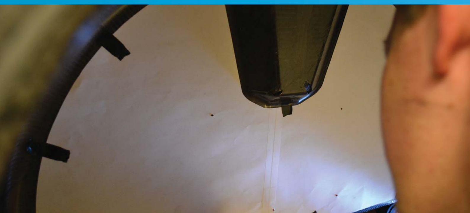
Paper template with the holes correct position in the rear wheel well
