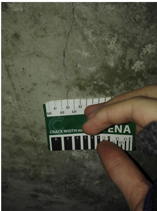
Figur 4.22: Riss innside brukasse
