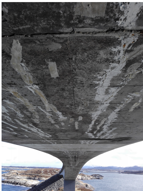
Figur 4.15: Riss i UK bruplate
