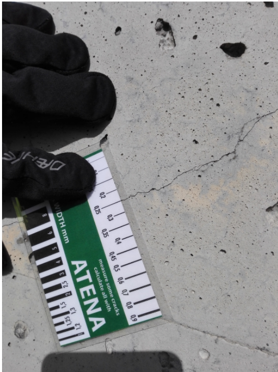
Figur 4.20: Riss i steg
