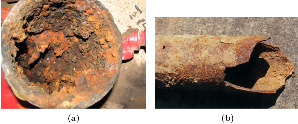
Figure 3.17: Corrosion damage in pipes. (a) Corrosion inside a pipe [Huguenot Laboratories, nd] . (b) Corrosion damage in a pipe has lead to a hole in the pipe [Colorado Geological Survey, nd].
