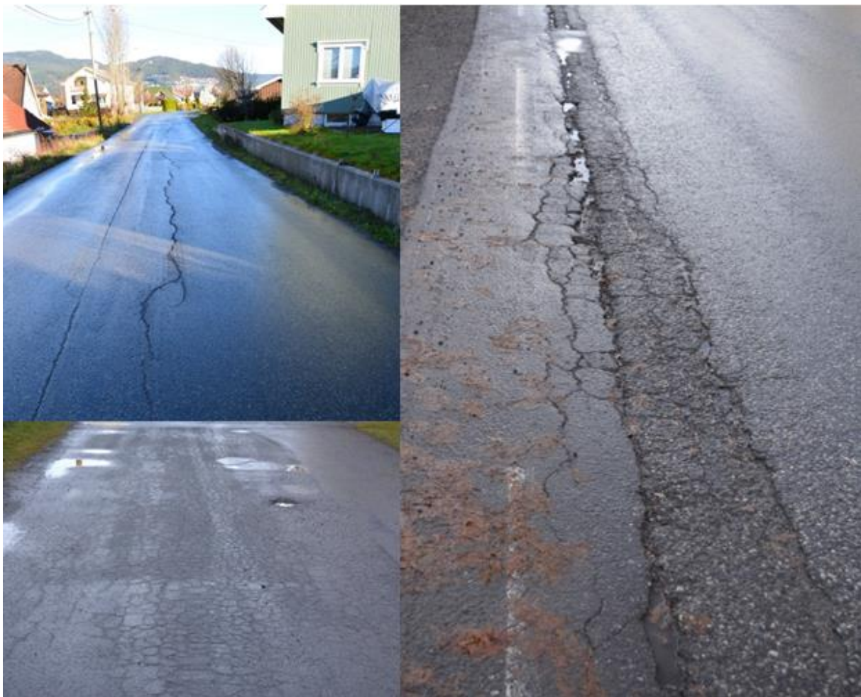
Figure 3:2 – Example of damages on an asphalt road (Photo: Erik Josepshon)
