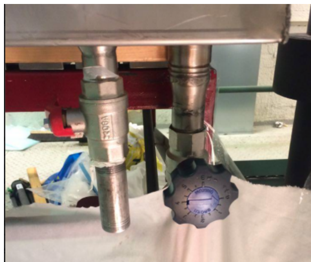
Figure 3.11: Draining valve (left) and downstream flow valve (right).
