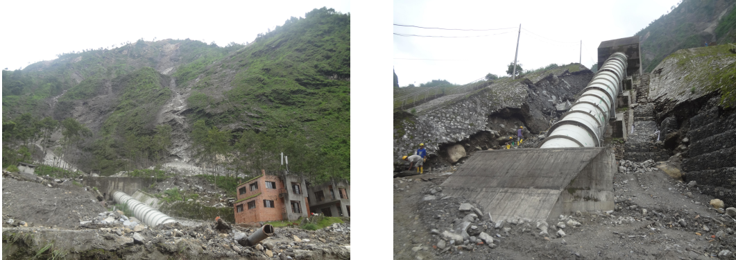
Figure 8.2: (LEFT) Penstock of Bhotekoshi HPP, which was burst due to the rockfalls from the cliffs in the background. (RIGHT) Scouring due to flooding after the penstock burst.
