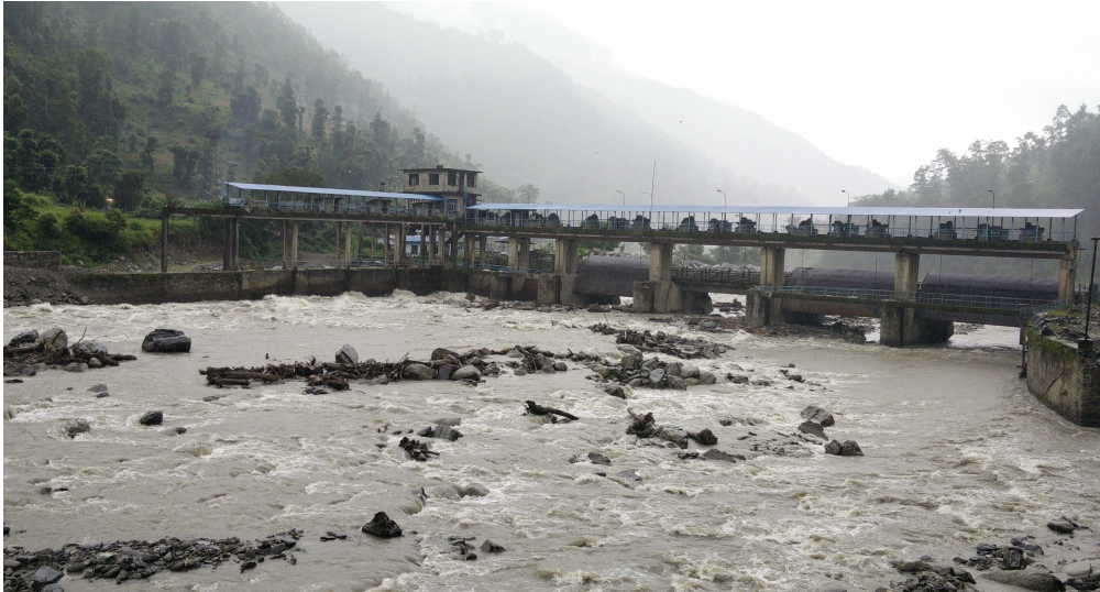
Figure 8.6: Intake of Sunkoshi HPP which bore the brunt of Jure rockslide as well as Gorkha Earthquake and the series of aftershocks.
