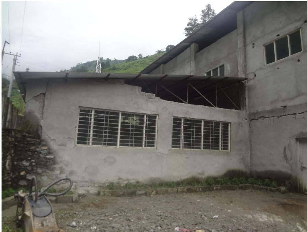
Figure 8.3: Cracks seen in the powerhouse of Middle Chaku HPP. The damages seen are mostly due to the shaking.
