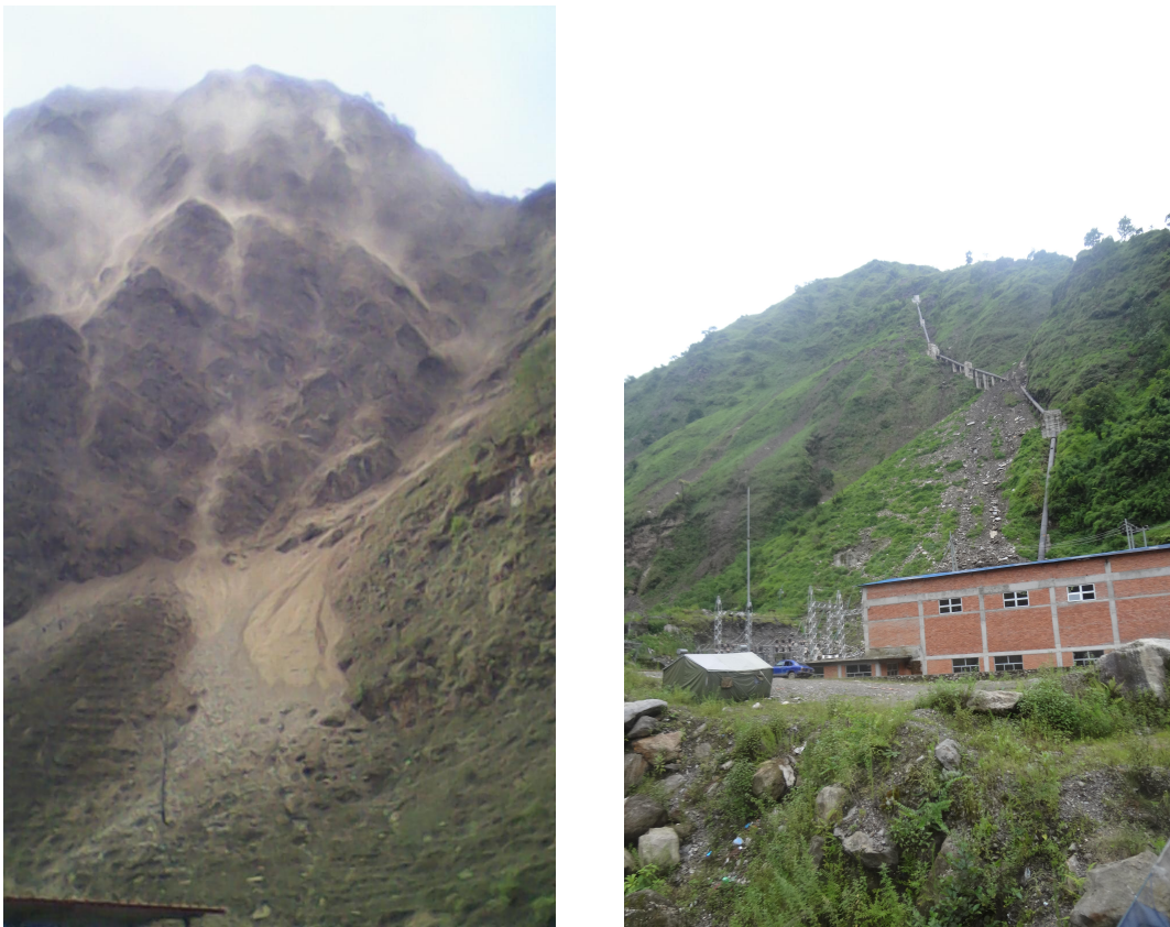
Figure 8.1: (LEFT) Debris fall in the intake area of Bhairabkunda HPP. (Photo Credit: Surya Thapa/Bhairabkunda HPP) (RIGHT) Penstock, powerhouse, and switchyard of Bhairabkunda HPP. The penstock and the switch yard were heavily damaged.
