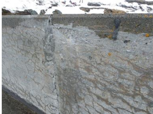
Figure 7.6: The typical map cracking pattern at Votna 1 (Photo: Gilles Plusquellec).
