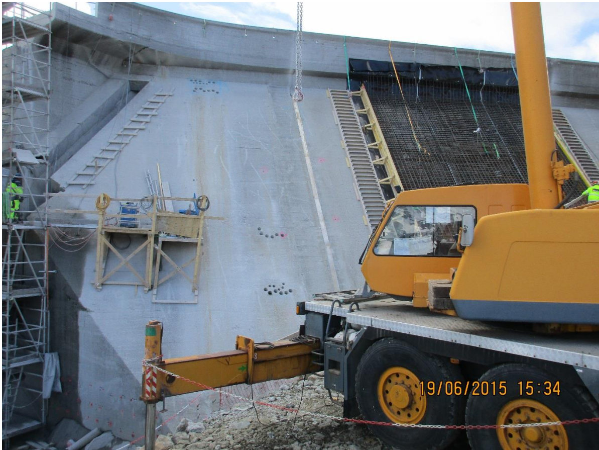
Figure 2.3: Slab dam after drilling (Provided by J. Lindgård).
