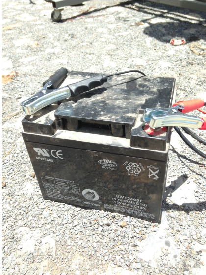
(a) Picture of the battery used to supply power to the pump.
