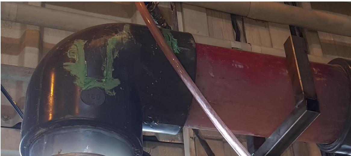
Figure 36 – Accumulation of oil at the outlet
