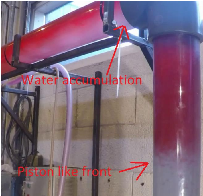
Figure 46 – Accumulation of water at bottom of first horizontal section ( 6\text{m}^3/\text{h} ).
