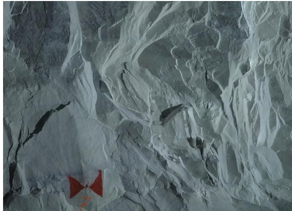
Figure 5.48: Loosened rocks stand out from the pillar’s surface
