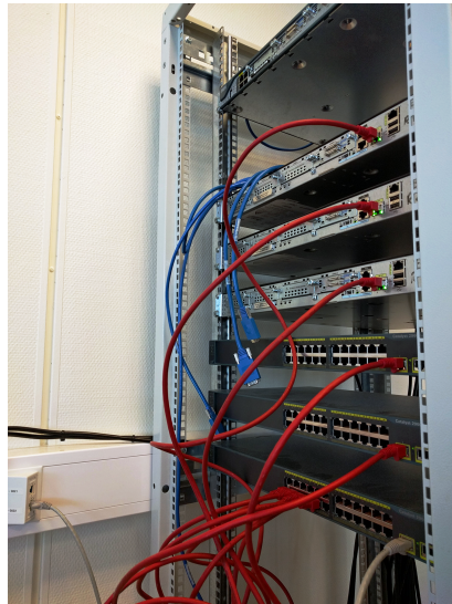
Figure 10: Cabling of equipment for test, the grey network cable is connected to GRANCONF, TFTP and DHCP server
