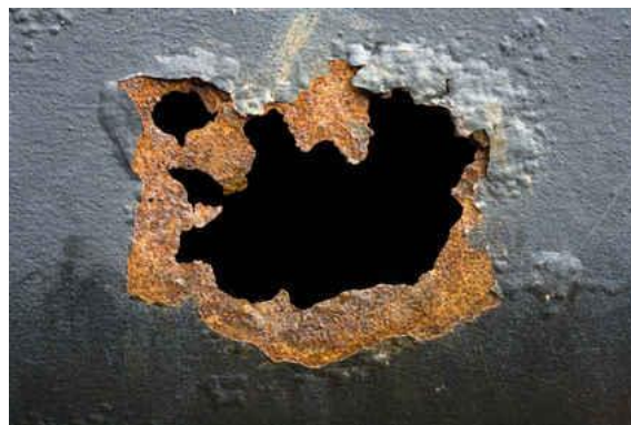
FIGURE 8 PIPELINE CORRODED (MERUS 2013).
