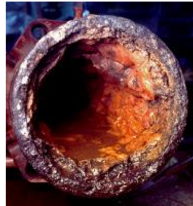
Figure 1.8 - Typical pipe with biofouling products
