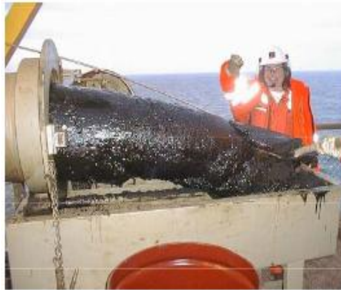
Figure 16. Wax plug removed through pigging (Time 2011)
