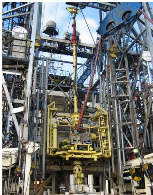
Figure 16: Derrick with SIL and TRT (Tree Running Tool) installed awaiting deployment [37]
