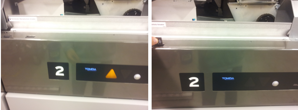
(a) The safety barrier is breached
