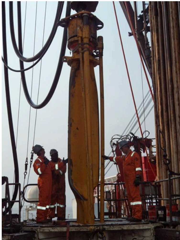
FIGURE 4: RISER COLLAPSE AT 1300 METRES (WWW.GCAPTAIN.COM, 2013)
