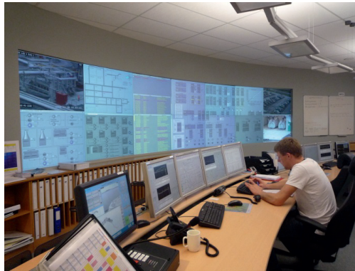
Figure 2-12: Control room at Shell's processing facility for Ormen Lange. (Photograph: author)
