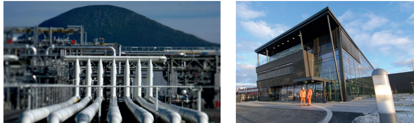
Figure 6-4: Left: Slug catcher where the process of separating gas and liquid starts. Right: Nyhamna's administration building. The building includes a simulator, a laboratory, a workshop, and the control room (Photographs: Shell).
