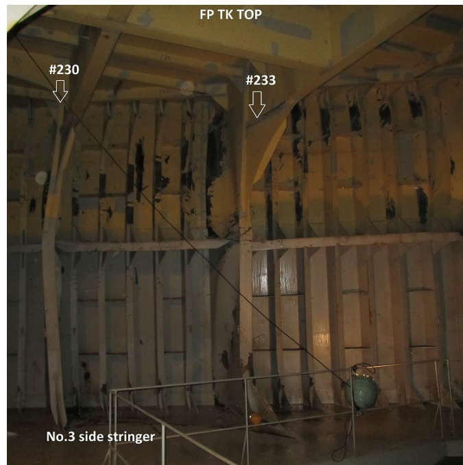
Figure 3.4: Indent seen from inside fore peak tank, [5]
