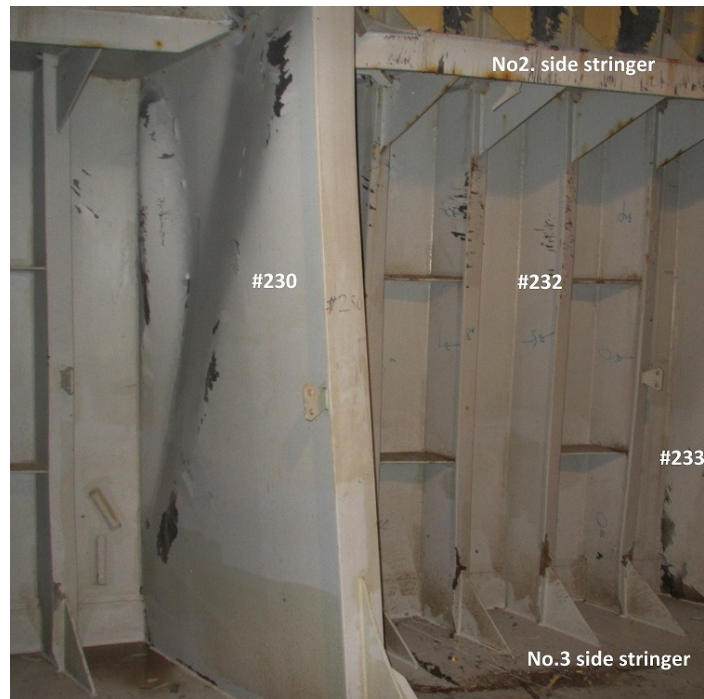
Figure 3.13: Deformation of frames and web frames #229 1/2 - #233, [5]
