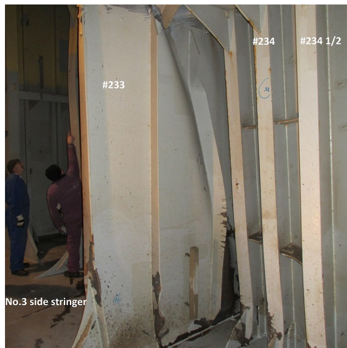
Figure 3.14: Deformation of frames and web frames #233 - #234 1/2, [5]
