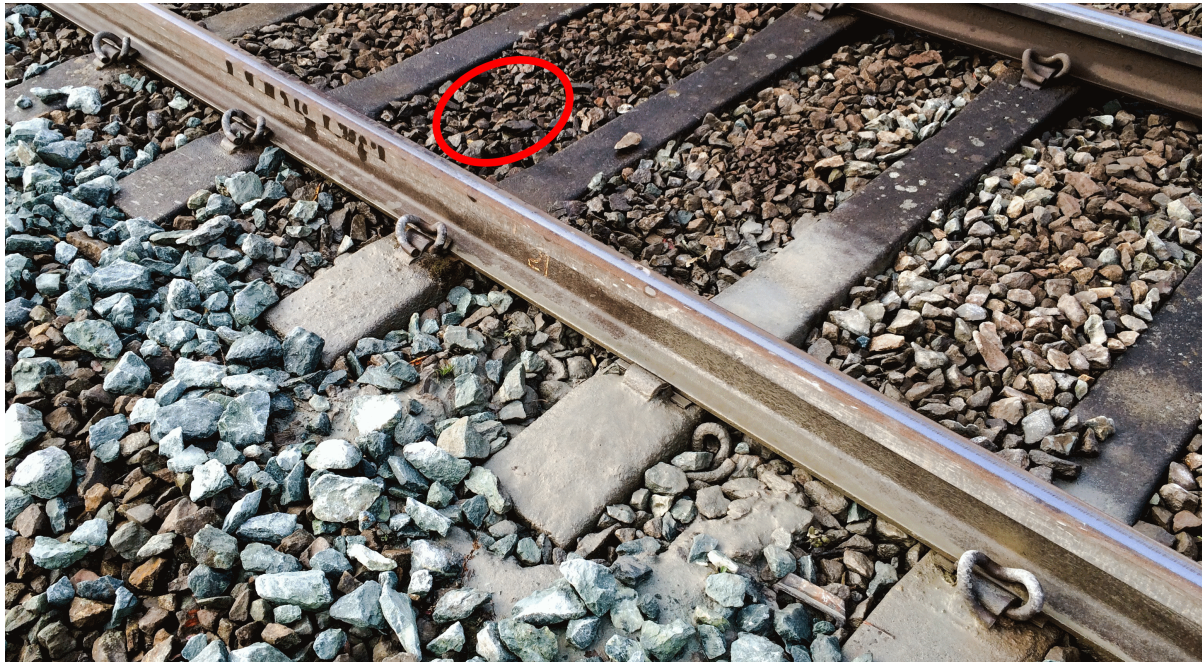
Figure 29: Water test site 2. Fines from mud pumping clearly visible on sleeper ends and adjacent ballast. Water was poured into the area marked in red.
