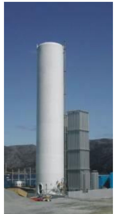
Figure 41. LNG satellite. Picture from [8]
