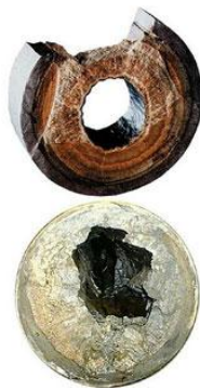
Figure 5:Scale in pipes
