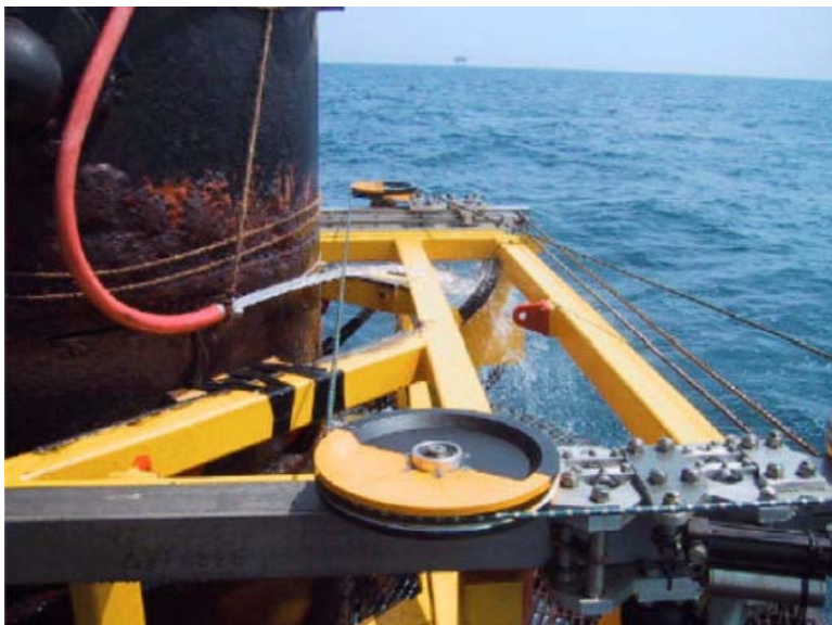
Figure 14: Illustration of diamond wire cutting of a deck leg, (Kaiser and Byrd 2005)
