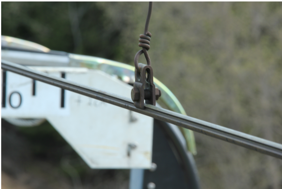
Figure 2.3: Dropper clamped onto the contact wire (Photo: Petter Røe Nåvik).
