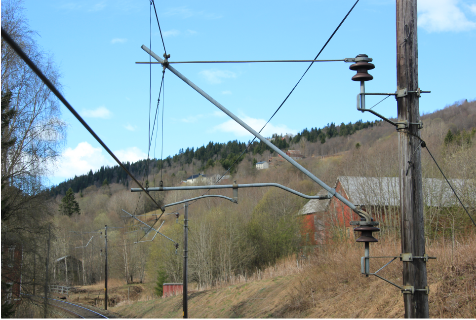
Figure 2.4: Support pole on a Norwegian track, part of the reference system (Photo: Petter Røe Nåvik).
