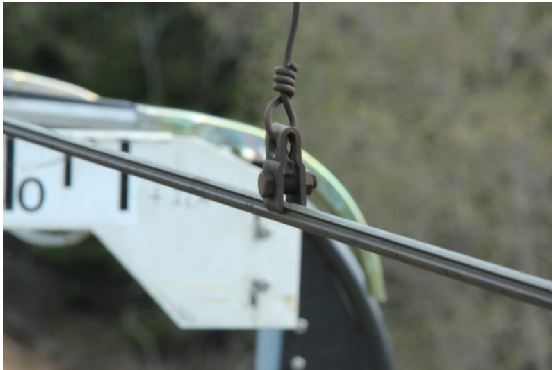
Figure 14 The dropper's connection to the contact wire at "Wire 152". The connection to the messenger wire is approximately the same.
