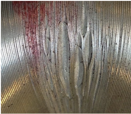
(b) Close-up of Pipe 1.
