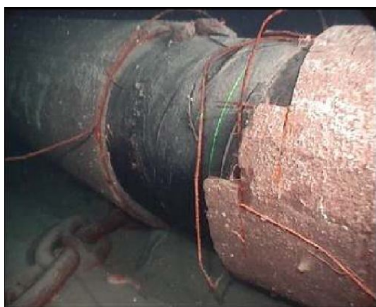
(a) Damaged pipeline
