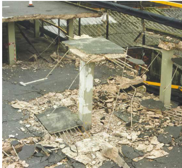
Figure 2.7: Global collapse of structure due to punching shear failure
