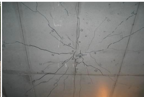
Figure 15: Slab 2 after testing (Døssland, 2008)
