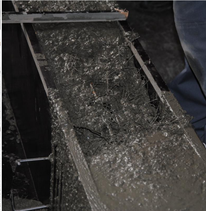
Figure 52: Lumping of steel fibres
