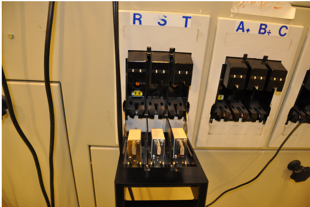
Figure F.9: Main fuse connecting laboratory circuit to the mains. 36 A fuses are used.
