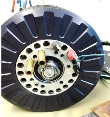
Figure A.4: Loose cable lug on PM motor phase.
