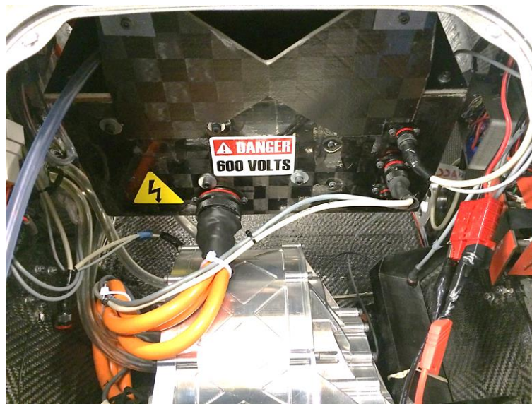
Figure 8.15: Motor room assembly, voltage source inverter and PM motor.
