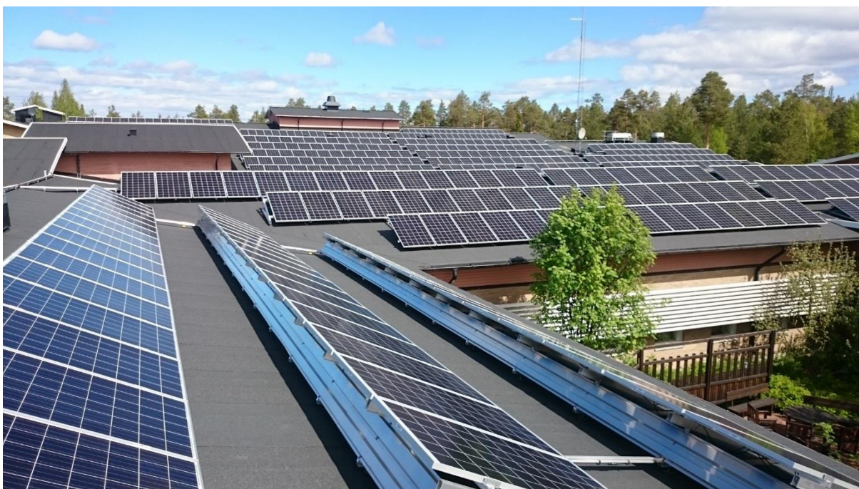
Figure 62 – Parts of the PV system at the Acusticum. Photo taken from roof I. Photo by Eirik Oksavik Lockertsen.
