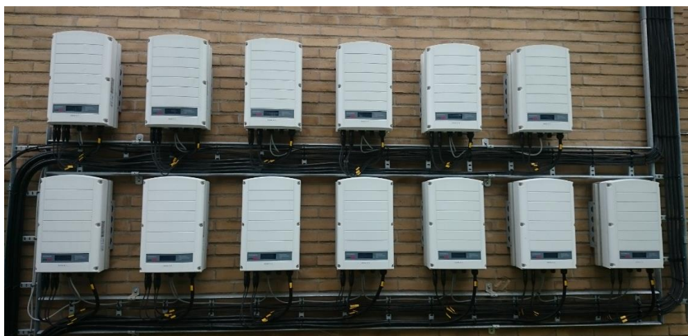
Figure 85 - The inverters at the Acusticum. Photo by Eirik Oksavik Lockertsen.
