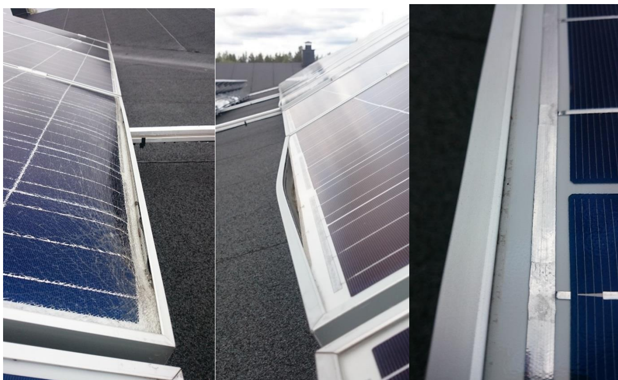
Figure 88 - Shattered, severely bent, and minor bent modules at the Acusticum PV system. Photos by Eirik Oksavik Lockertsen.
