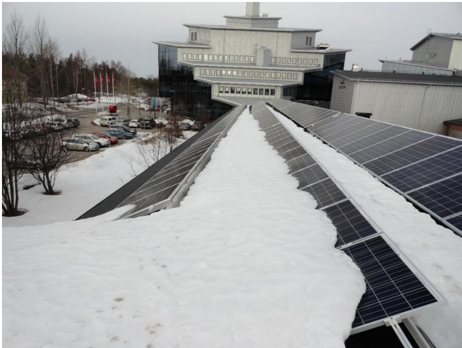
Figure 89 – Snow covering PV modules at roof A. The shattered module is the 4 th in the middle row. Shot at 27 th of March 2015. Photo by Øystein Kleven.
