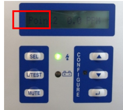
Figure 3-7: Gas alarm system monitor
