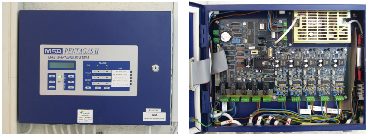
Figure 3-6: Overview of the Gas warning system (External and Internal views)
