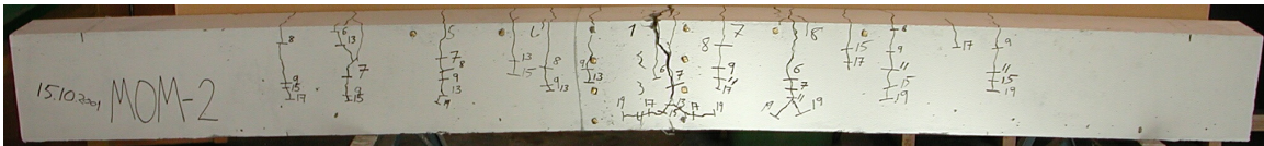
Figure 6.9: Cracks in beam M2-A; average crack distance 123mm. The cracks were traced with a marker for each load-step.
