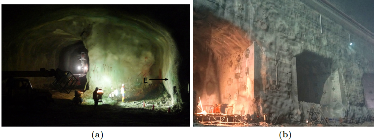
Figure 4.16.: (a) Squeezing in pillar wall. (b) Concrete jacket installed for niche pillar. Photos byNorplan A/S (2013b).
