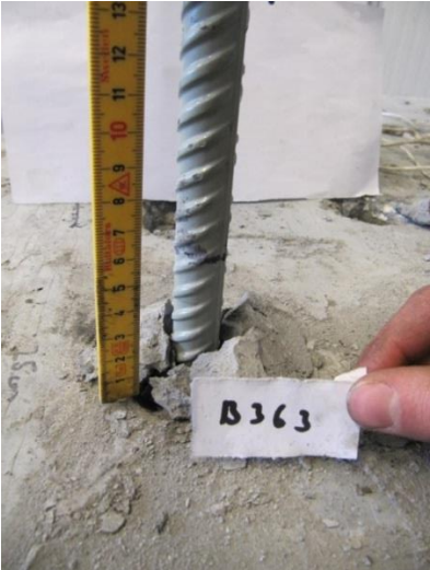
Figure 53 – Pull out length is 5.5 cm and the grout has broken in the surface. This bolt yielded before it slid from the grout.
