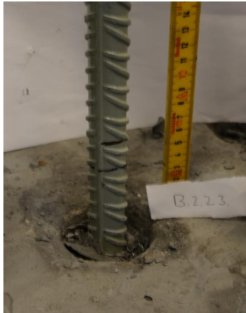
Figure 43 – Pull-out length is 6 cm. This bolt yielded before it slid from the grout. The figure shows how the surface of the grout breaks around the bolt.
