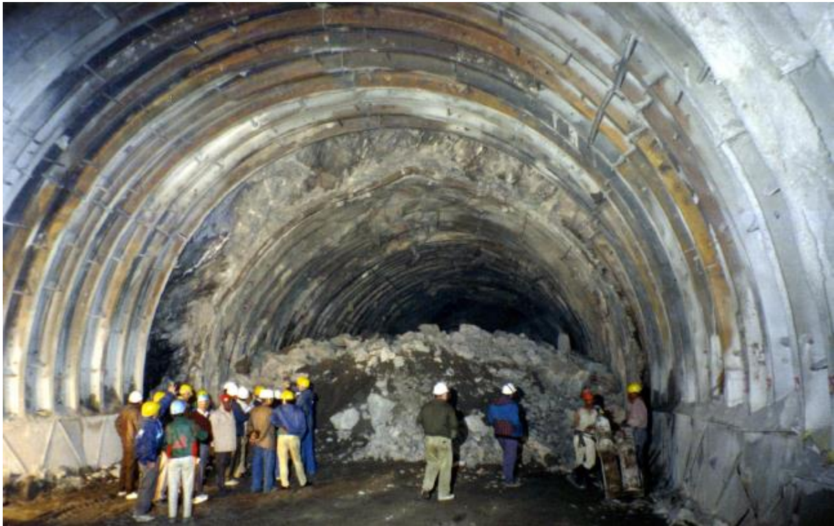
Figure 20 – Squeezing in a 10 meter span tunnel. Approximately 1 meter of inward displacement is in the roof and sidewalls (Hoek and Marion. 2000).
