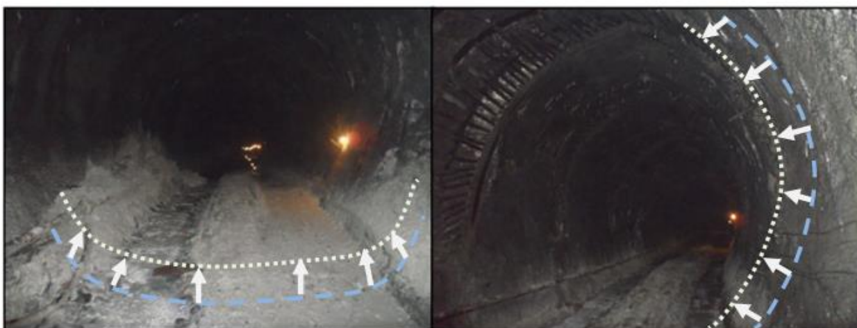
Figure 4-9: Tunnel squeezing in headrace tunnel of CHEP: Significant floor heave (left) and wall closure in hill side (right)
