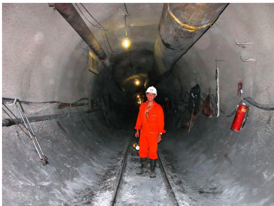
Figure 5-15: Completed tunnel lining in one of the deepest sections between Chainages 10000 and 12000 in Yacambú-Quibor tunnel (Hoek and Guevara, 2009a)
