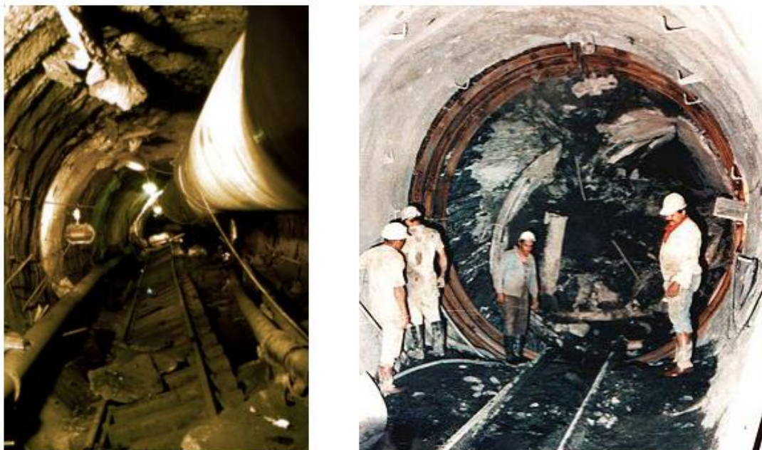
Figure 5-10: Floor heave about 100m behind the Intake drive TBM in 1979 at a depth of 400 to 425 m below surface (Hoek and Guevara, 2009a) (left) and Mining out the remains of a tunnel boring machine trapped by squeezing of the tunnel during a stoppage of the drive (Hoek, 2001) (right).
