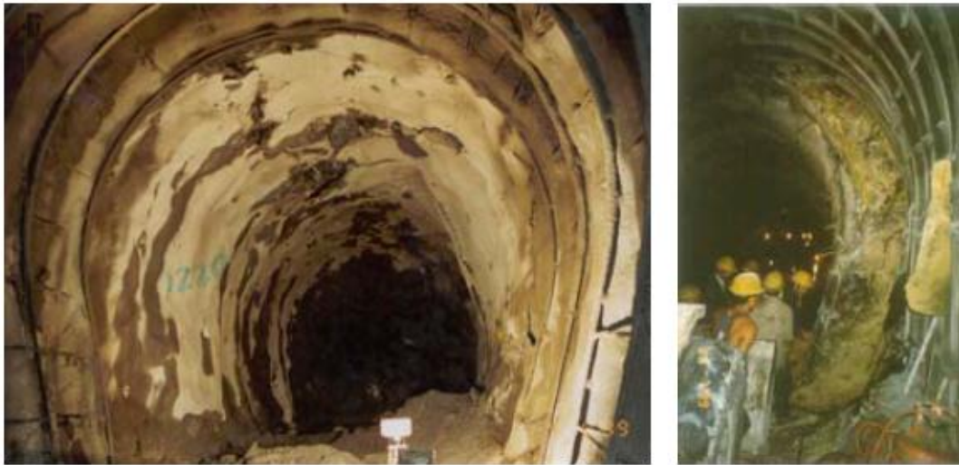
Figure 5-13 : Squeezing in tunnel kaligandaki HEP (left) and Modi (HEP) right. (Panthi 2000) Some Prediction for tunnel Squeezing based on empirical and semi analytical approach has described below.
