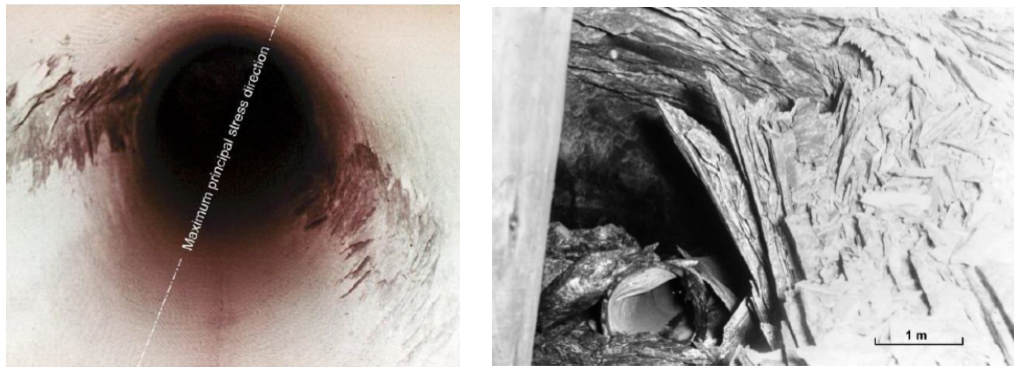
(a) Brittle failure in the walls of a bored vertical shaft in a hard rock deep mine (b) Result of a rockburst in a deep level gold mine in South Africa
