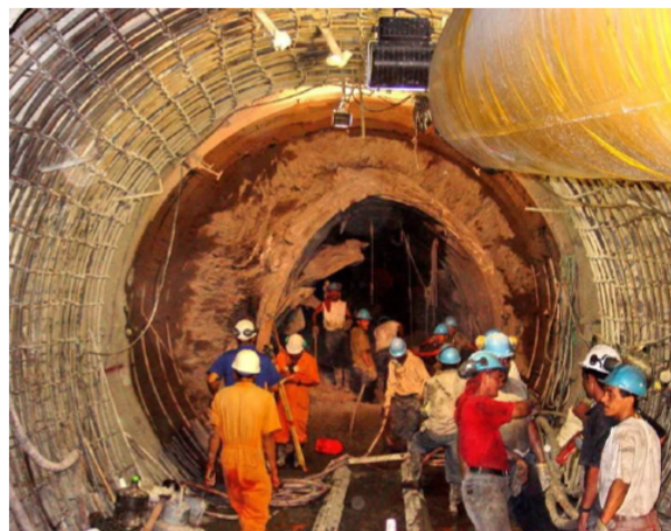
Figure 28: Failure of a tunnel section due to very severe squeezing (background) and re-mined and re-supported tunnel (foreground) (Hoek & Marinos 2009).
