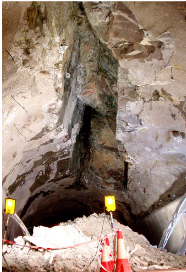
Figure 26: Image from rock fall in the Hanekleiv tunnel. The rock fall was caused by a weakness zone containing swelling clay (Picture in courtesy of Statens Vegvesen).
