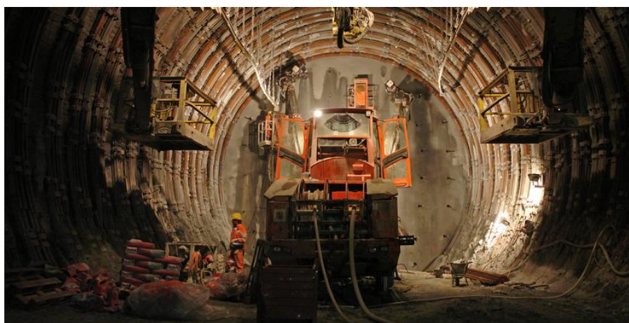
Figure 20: Excavation at the Sedrun section using drill and blast. Here, the main tubes were supported by a tight pattern of steel arches (AlpTransit Gotthard Ltd 2012).
