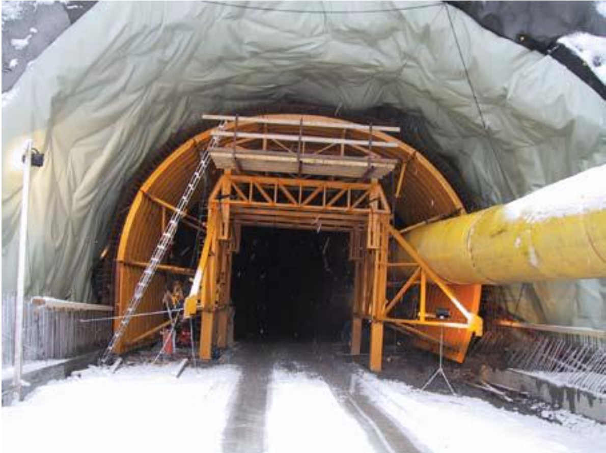
Figure 32. A shield used for concrete lining in the entrance tunnel to the Melkøya tunnel. (Sve, Elvøy et al. 2008)
