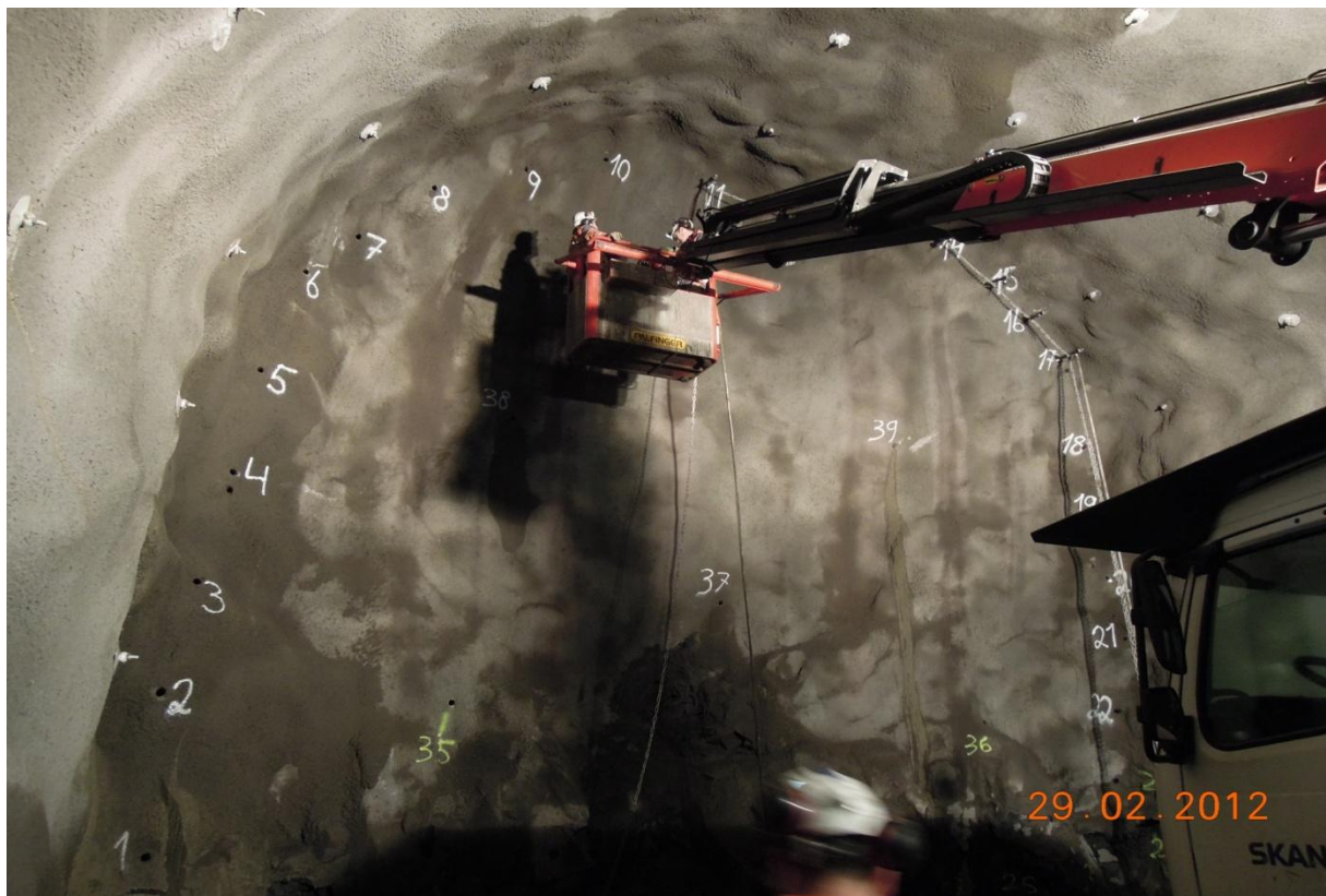
Figure 27. Grouting rods being inserted at the tunnel face in the R7 entrance tunnel.
