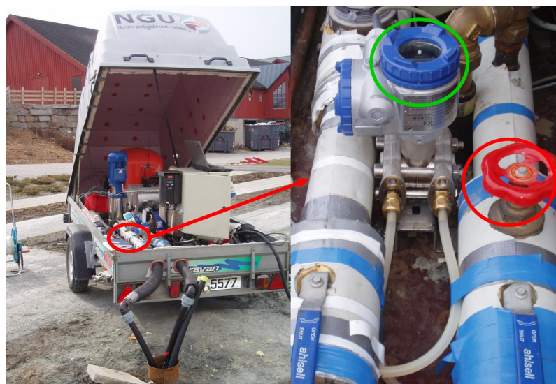
Figure 3.6: Thermal response test rig (left) showing the location of the differential pressure transmitter (right - green circle) and restriction valve (right - red circle). Photo: Marie Stølen
