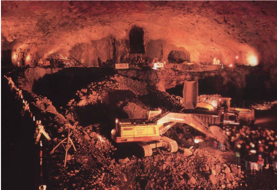
FIGURE 5.4 Photo from the construction of the Gjøvik Olympic Mountain Hall (from the research program “Rock Cavern Studium“, 1992)
