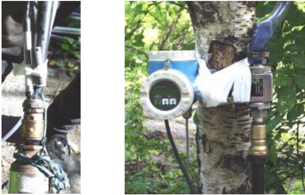
Figure 2–22: Pressure sensor connected to the test pumping equipment (left), and a flow meter (right).
