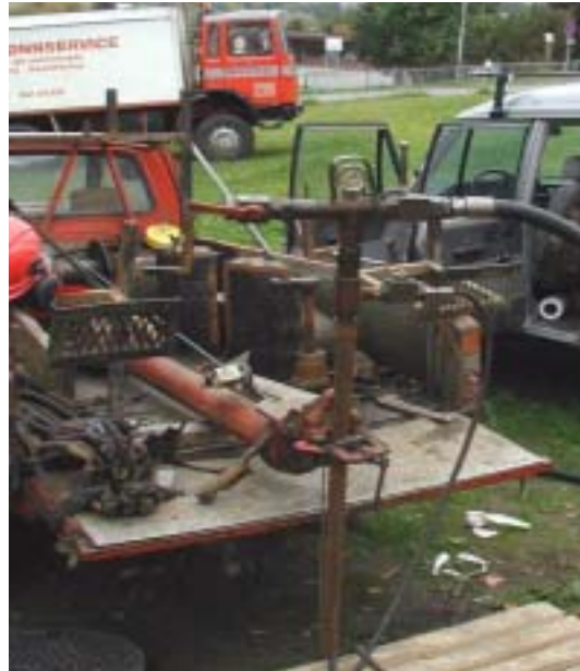
Figure 2–9: A T-coupling unit on top of the downhole equipment for hydraulic fracturing where a high pressure water hose from the tank lorry is connected. The hydraulic hose below the water hose is for the measurement of water pressure.
