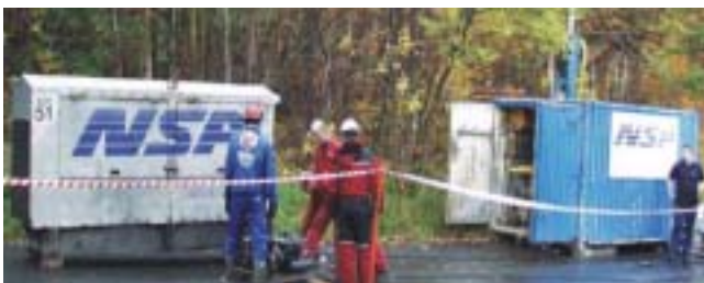
Figure 4-5: A mobile power supply equipment and the mixer-, container- and injection pump unit. The Hafo 2000 drilling rig is in the background.
