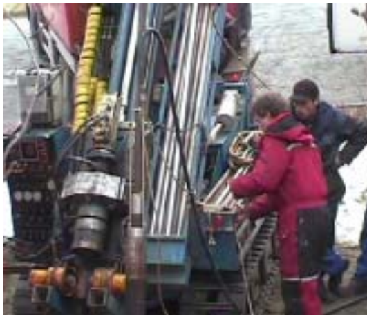
Figure 4-3: Lowering the double packer into borehole 1 at Lade using a Hafo drilling rig.
