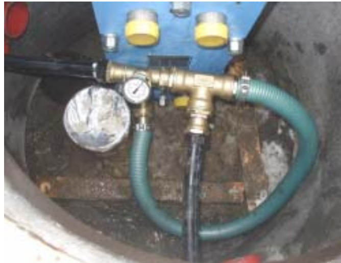
Figure 4–22: The heat exchanger in the manhole around the top of borehole 1 at EAB. The inflowing groundwater from borehole 2 and 3 are connected through a T-coupling to the heat exchanger. The outflowing water will be reinjected into the groundwater magazine via borehole 1 (on the picture). The in- and out collectors of the TRT-unit will be connected to the two upper exits, with yellow caps, on the heat exchanger. The system pressure is monitored by an analog manometer.
