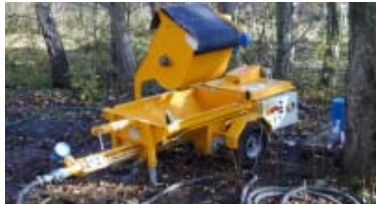
Figure 4–10: Mixer- and pumping unit.
