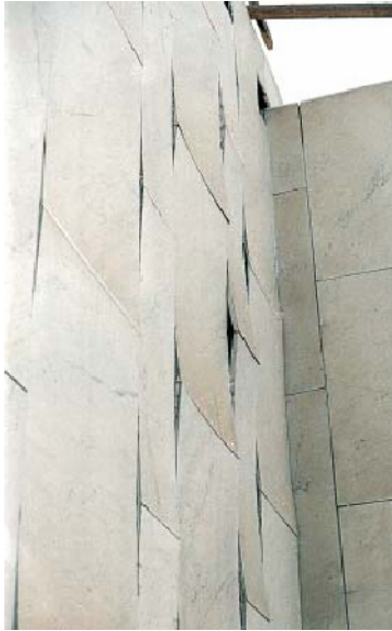
Figure 1. Warping marble cladding panels at the Finlandia Hall, Helsinki. Photo: TEAM project.
