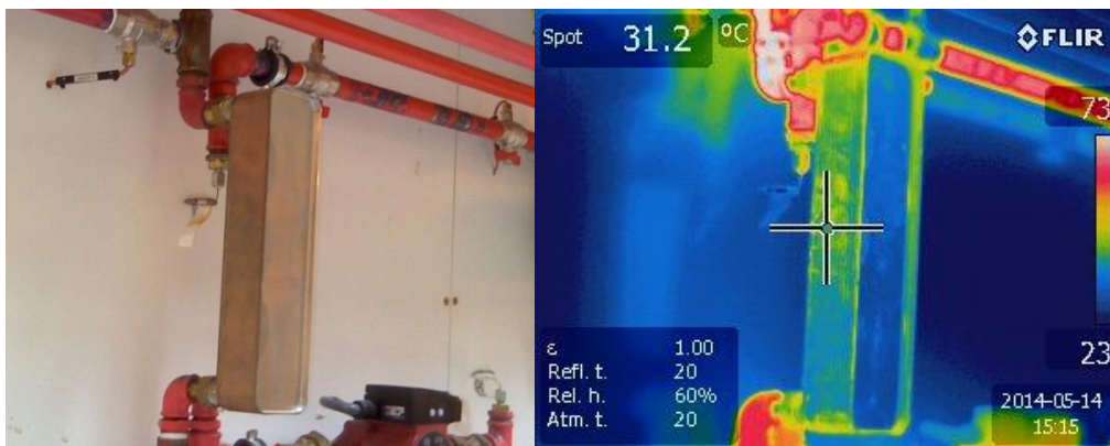
Figure 3.9 Picture and infrared capture of the HEX1 in operation
