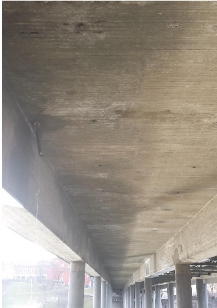
Figure 6.3: Visible moisture level differences on the bridge deck.
