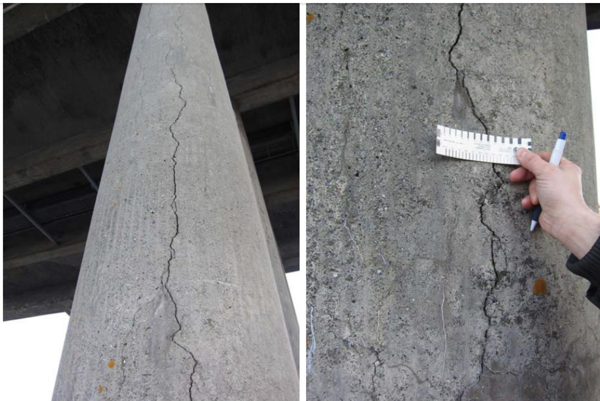
Figure 4.4: Pictures of the crack pattern, from NCAL's inspection and report on the columns.
