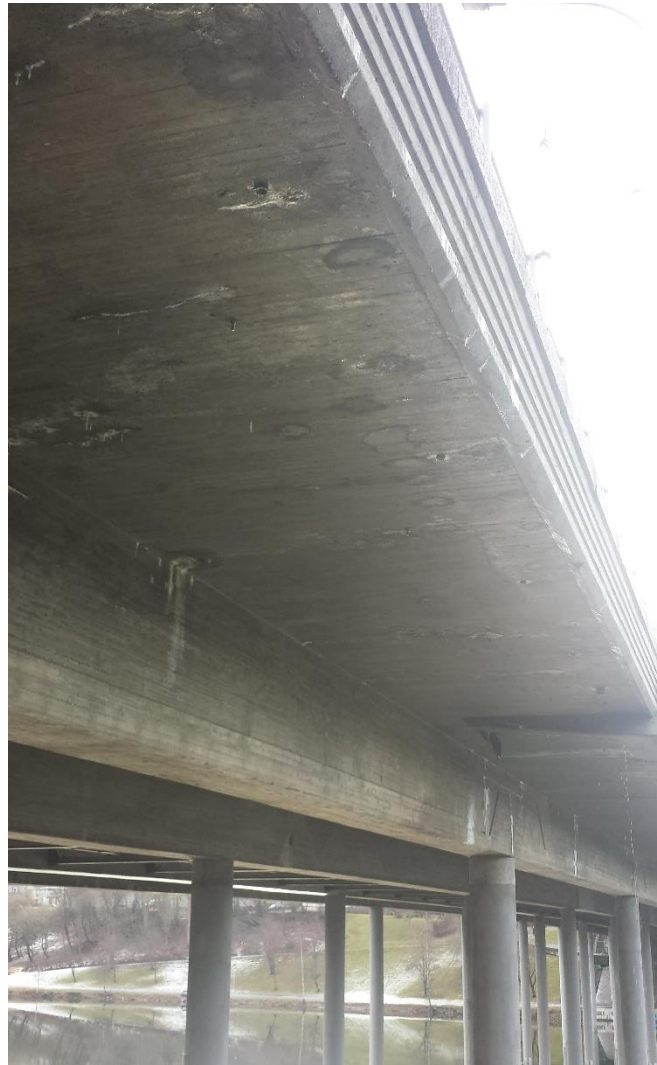
Figure 3.2: Some structural effects and damages on Elgeseter Bridge.
