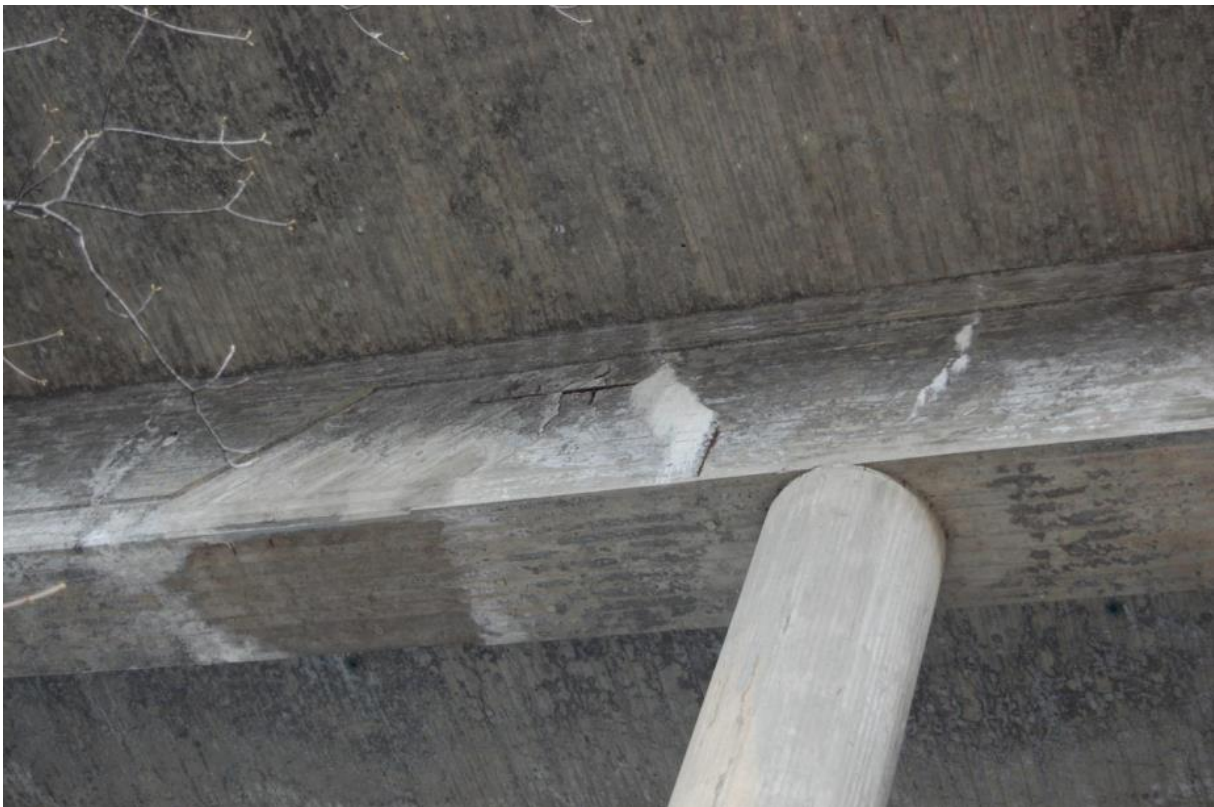
Figure 3.4: DEF and ASR occurring in Elgeseter Bridge.
