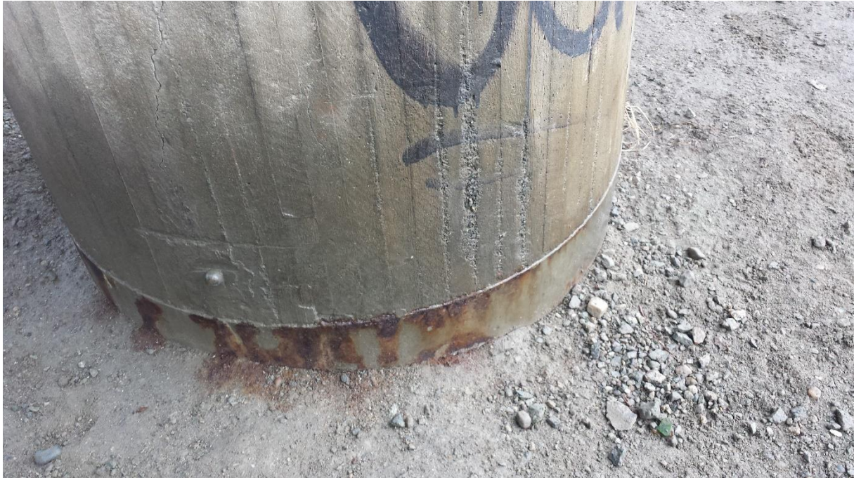
Figure 3.3: Refurbished column still shows sign of earlier combination of ASR and corrosion of reinforcement in the excess rust at the bottom.
