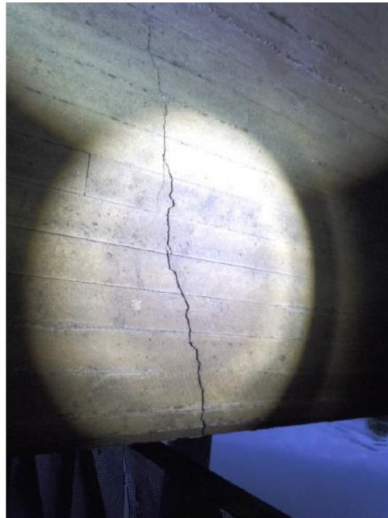
Figure 4.5: Picture of the vertical crack in span 8-9 from Rambøll's report from 2011.
