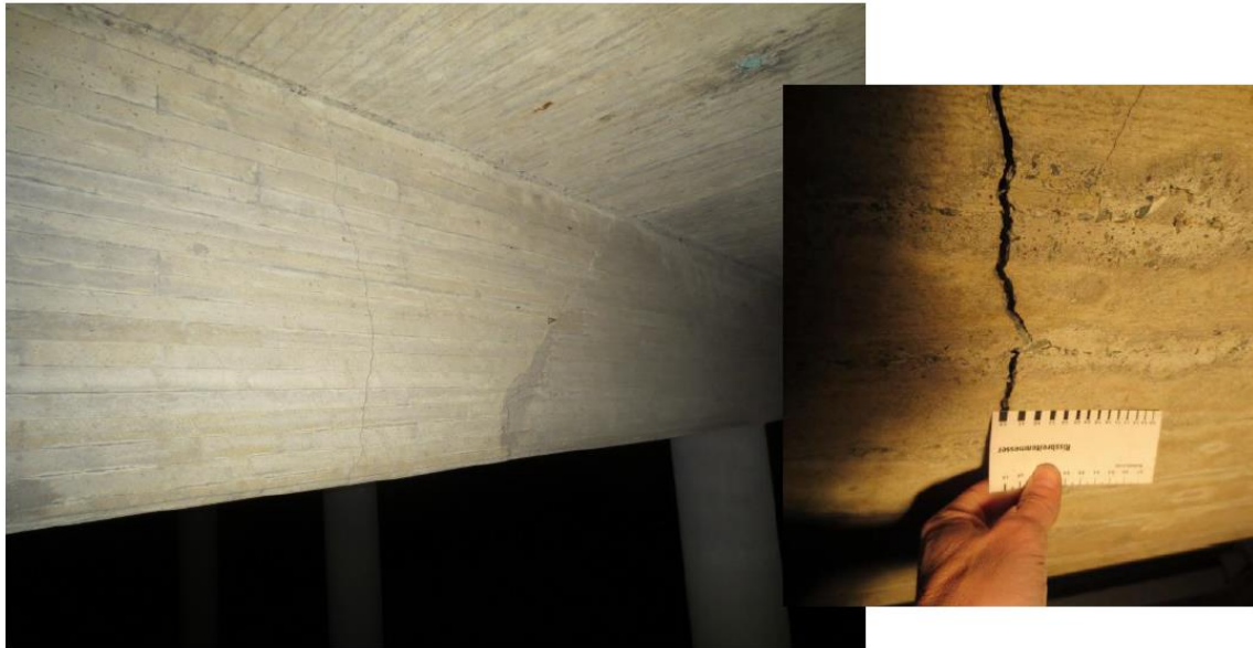
Figure 10.1: Pictures of the large crack in span 8-9, taken by Aas-Jakobsen [9].
