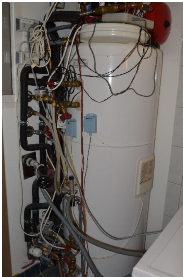
Figure 34: Image of the customized storage tank and the hydraulic connections
