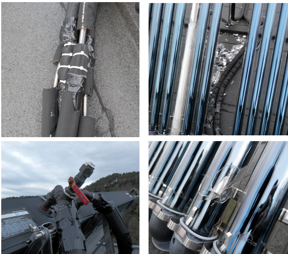
Figure 33: Pictures taken of the solar thermal systems at Løvåshagen. Top and bottom left: Incomplete insulation of pipes and connections. Top and bottom right: Broken collector tubes. Photos: Magnar Berge
