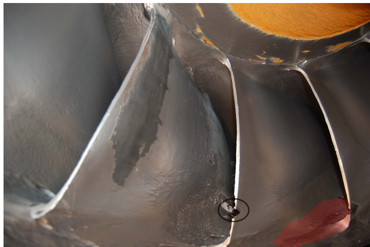
Figure 4.5: Erosion at runner outlet, Cahua power plant
