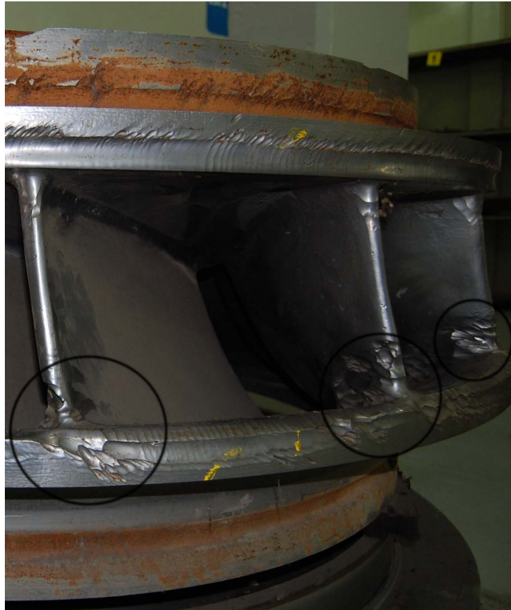
Figure 4.4: Old runner, Cahua power plant
