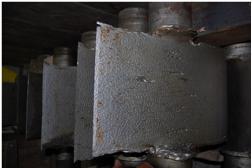
Figure 4.2: Eroded guide vanes, Cahua power plant
