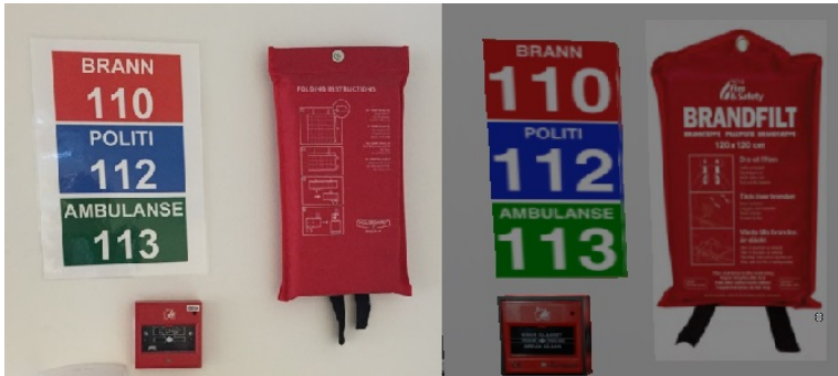
Figure 4.15: Emergency information, fire blanket and alarm button in the real location and in the virtual office.
